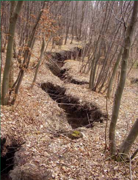
Subsidence cracks on slopes adjacent to the reservoir (Photo by O. Vasyliuk)
